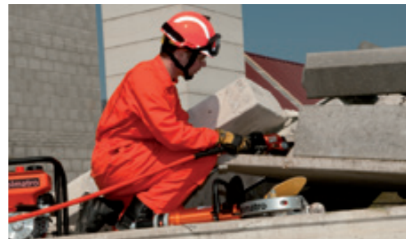
A perfect combination: crushing concrete with the CC 23 and cutting re-bar with mini cutter CU 4007 C or SMC 5006
